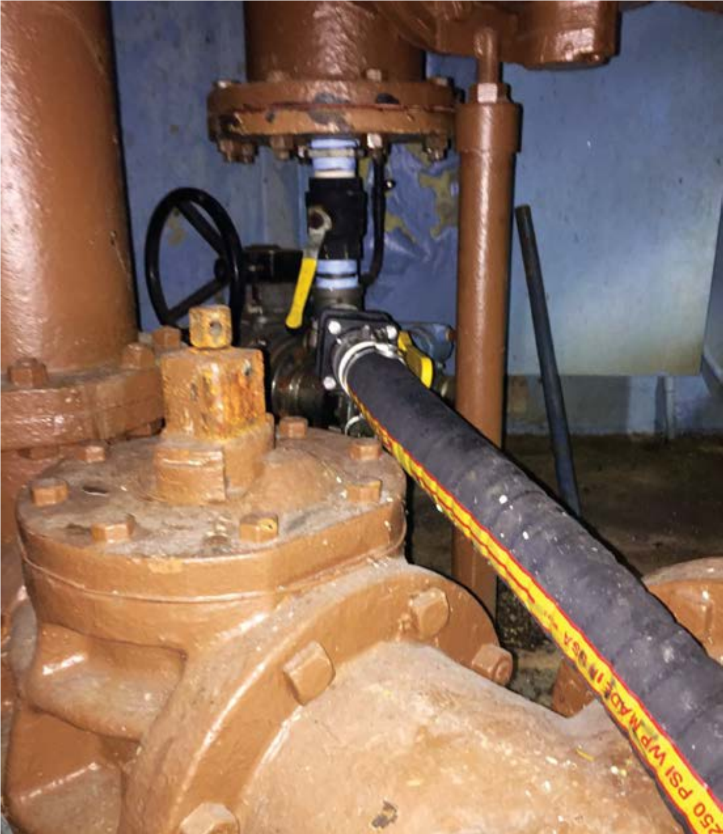
The chemical-based process for removing struvite in pipe has been successful for the Bethlehem Wastewater Treatment Plant's internal distribution lines.
