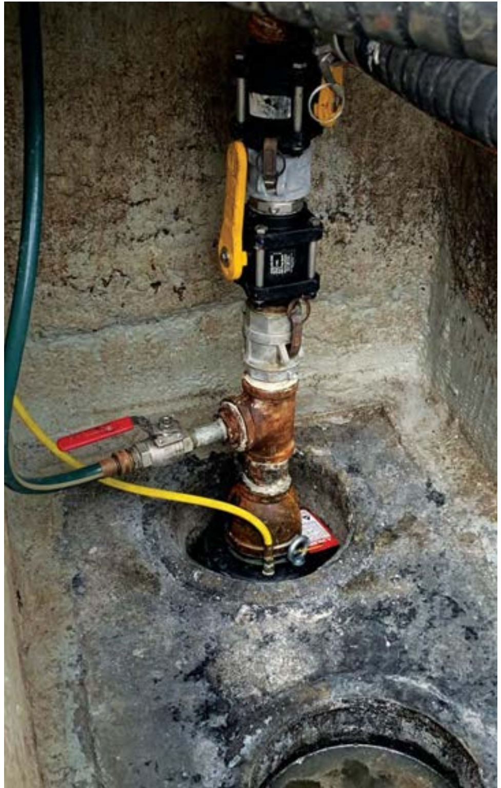
Struvite is a crystalline structure of magnesium, ammonium and phosphate that commonly builds up in pipe networks and is resistant to traditional maintenance methods for removal.
