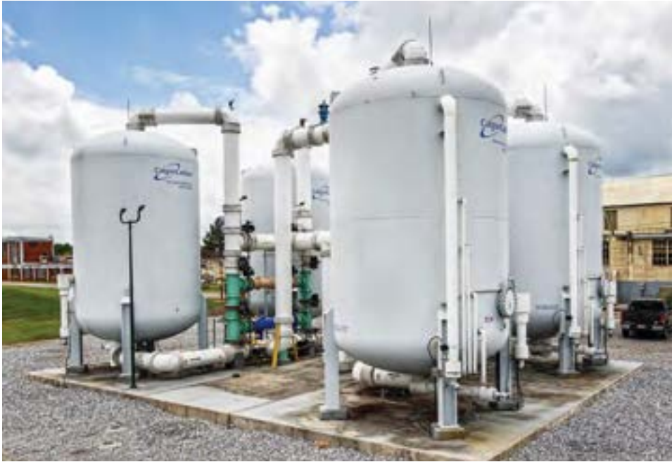
Shelby County Water Services selected granular activated carbon vessels that hold 60,000 pounds of granular activated carbon each to treat its water and comply with U.S. EPA Stage 2 DBPR standards
