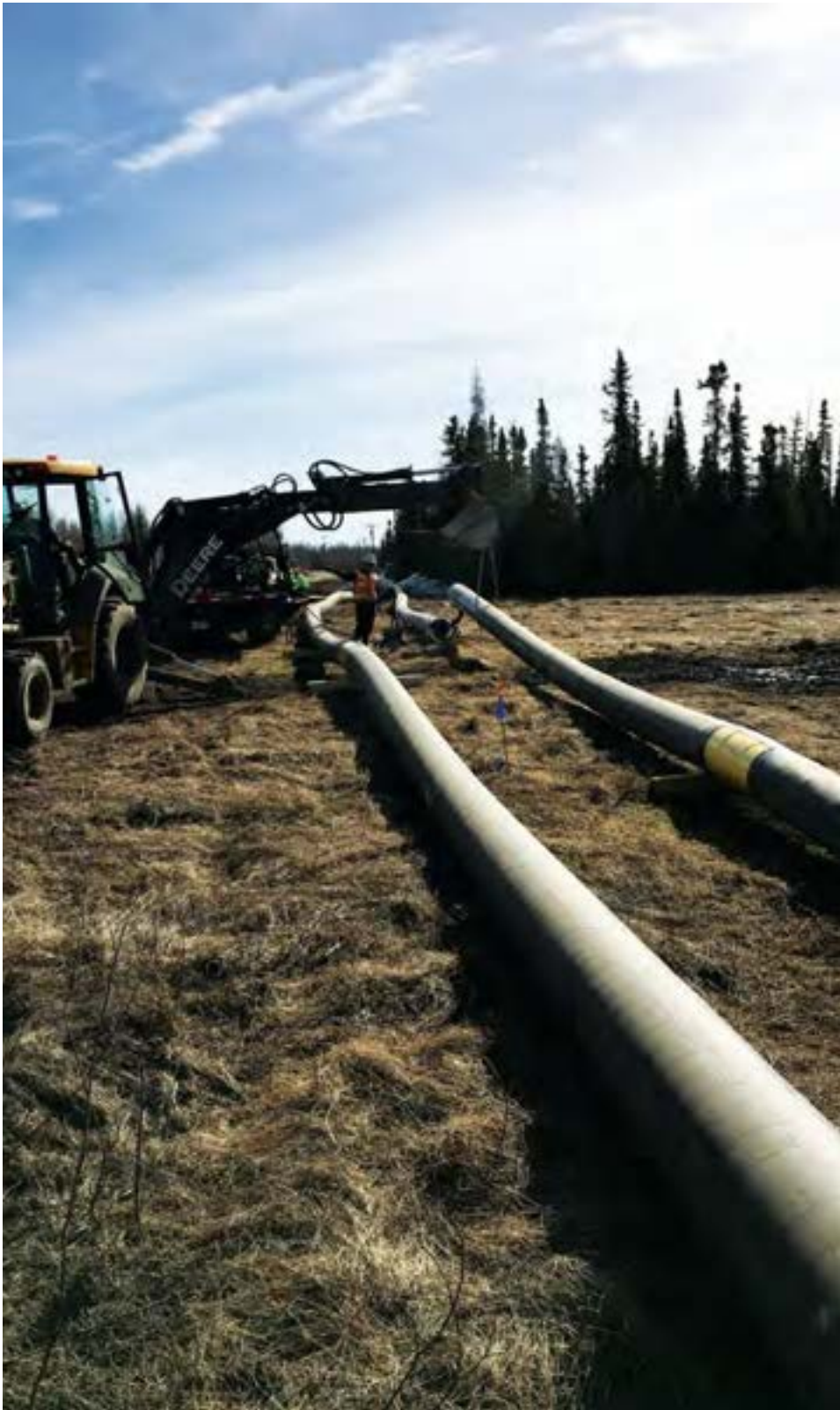
To provide a reliable water source for North Pole, Alaska, the city installed 35 miles of pipe as well as a 750,000-gallon reservoir totalling $52.1 million.
