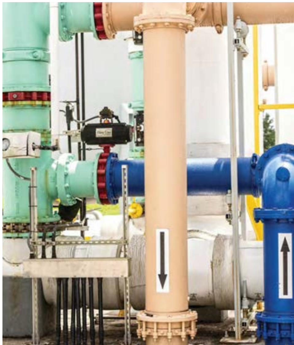
Not only is granular activated carbon effective at removing disinfection byproducts, but it also removes natural organic matter, pesticides and perfluorinated compounds.
