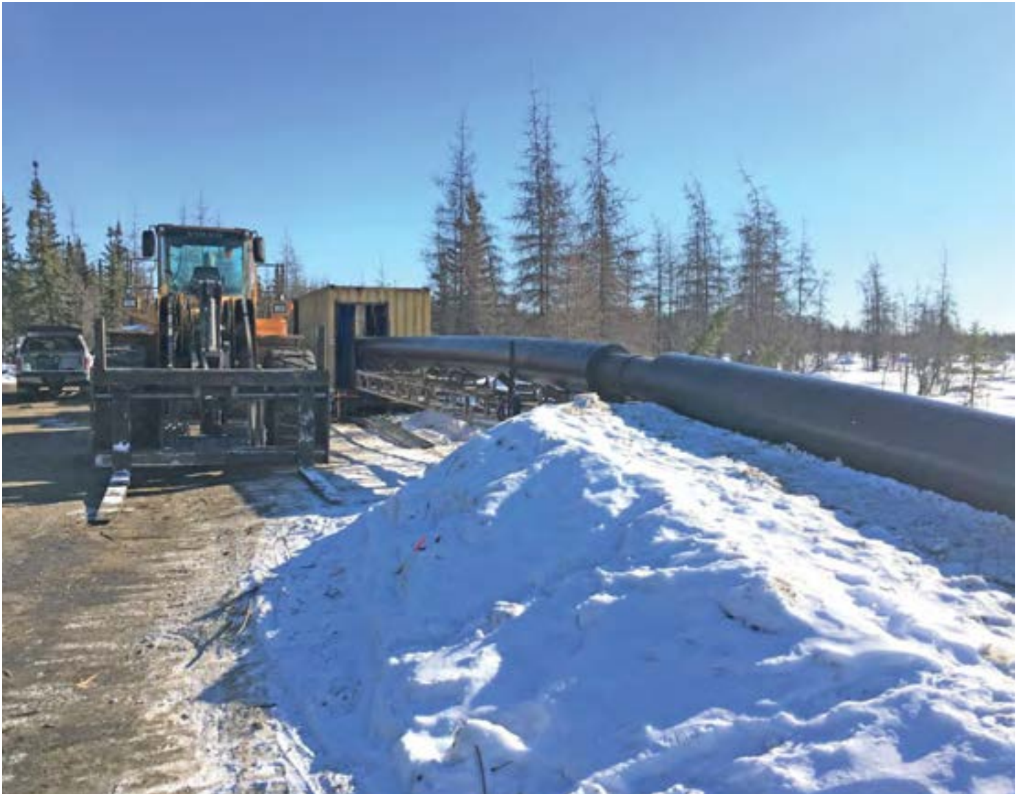
To accommodate freezing conditions, workers wrapped in a 3-inch insulation jacket around the high-density polyethylene pipe installed in North Pole, Alaska. Seismic activity also is a regular occurrence and despite more than 200 quakes registering 1.5 magnitude or greater, the pipe continues to function as intended.
